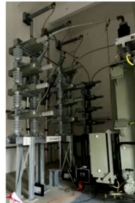
Indoor application: RC-Tower and shunt reactor
