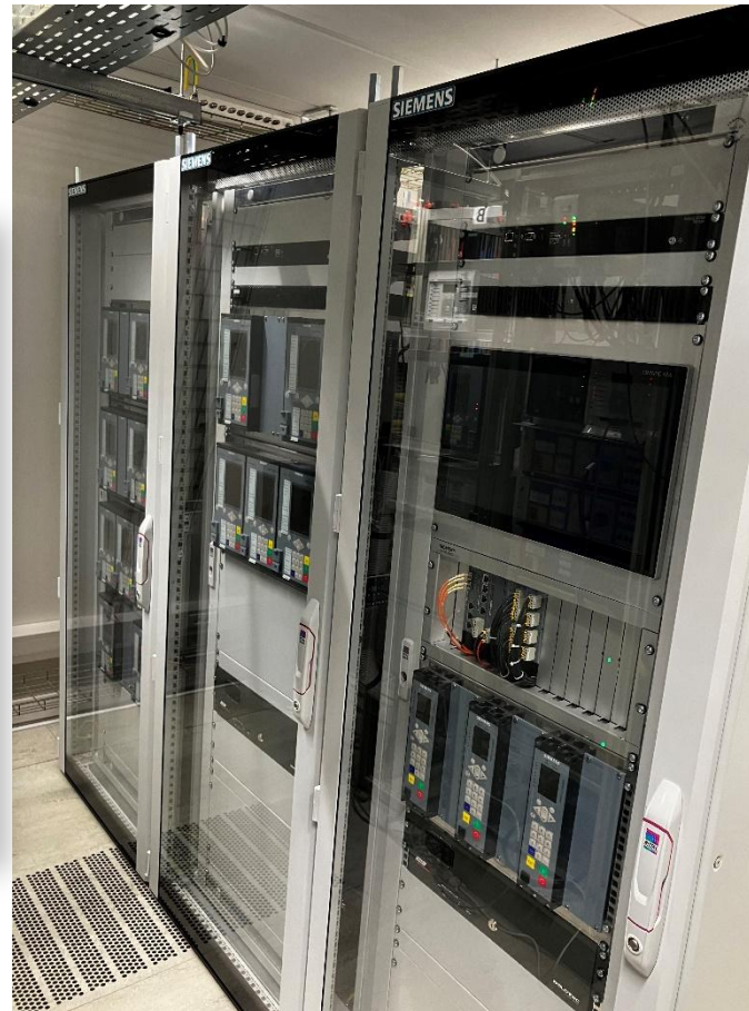
TU Delft Digital Substation (150 kV / 10 kV)
