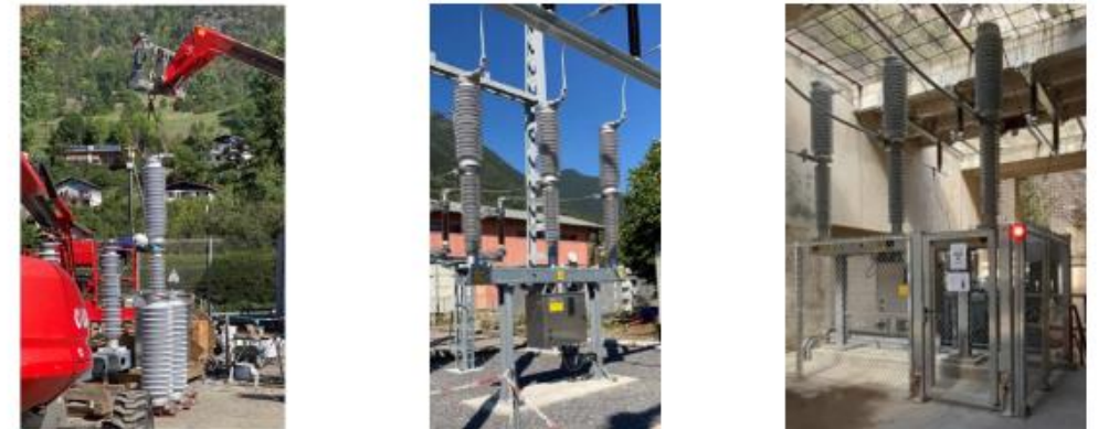
Figure 7: On-site assembly of the interrupter unit (left), CB inside a standard substation (middle) and CB inside an indoor substation (right)
