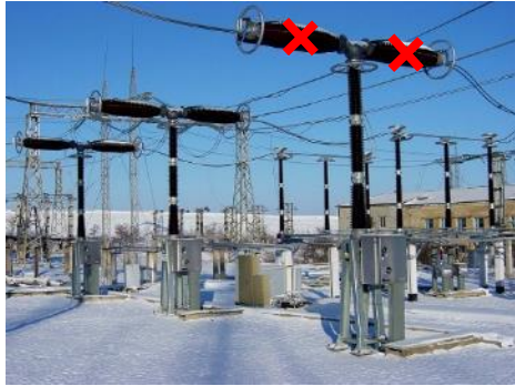
live tank circuit breaker (LT)
