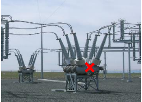
dead tank circuit breaker (DT)
