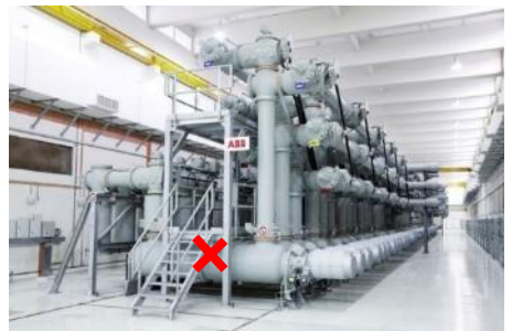
GIS circuit breaker
