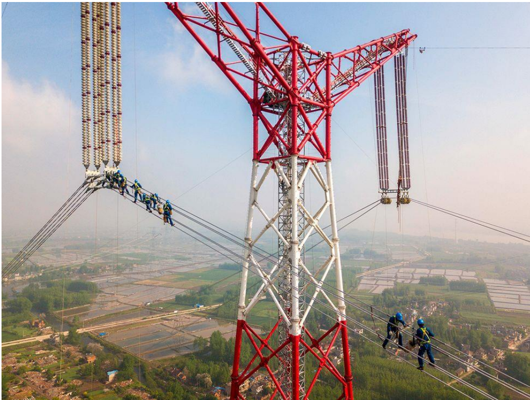
Laborers work on the construction of the Changji-Guquan ultrahigh-voltage direct-current transmission link along the Yangtze River, in Anhui province, China, in 2018.
